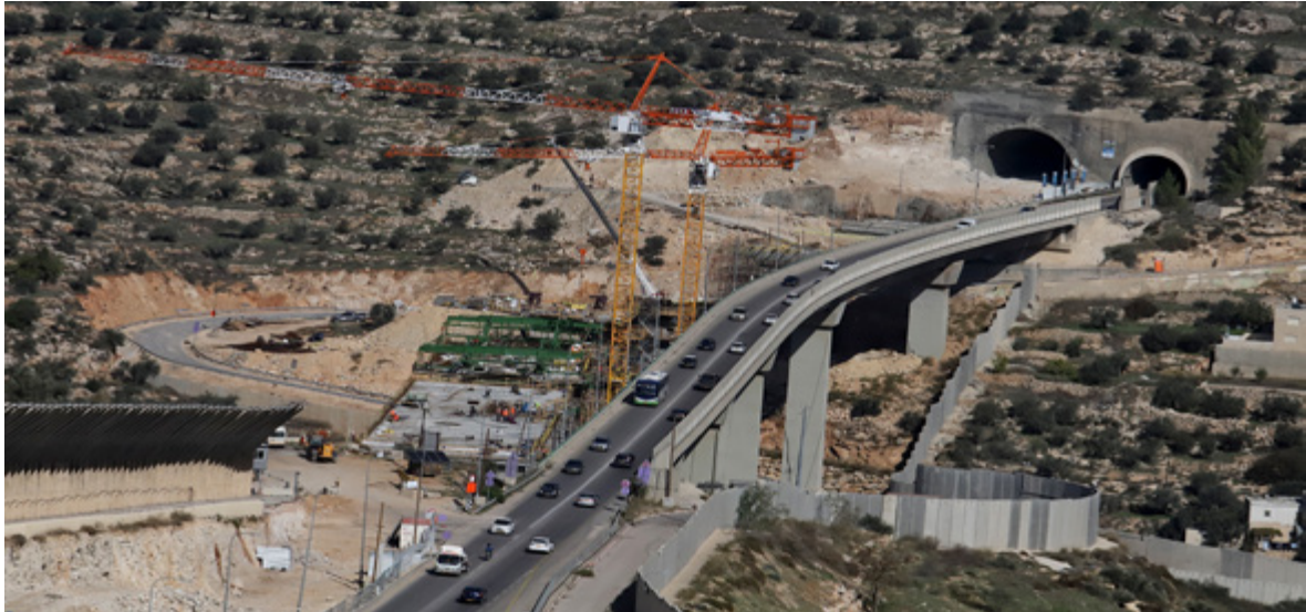
Construction to double the width of the Bethlehem Bypass Road (Highway 60 / the Tunnels Road)
